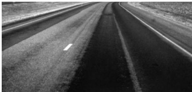
Gambar II.9 Contoh Jenis Kerusakan Utility Cut Depression
